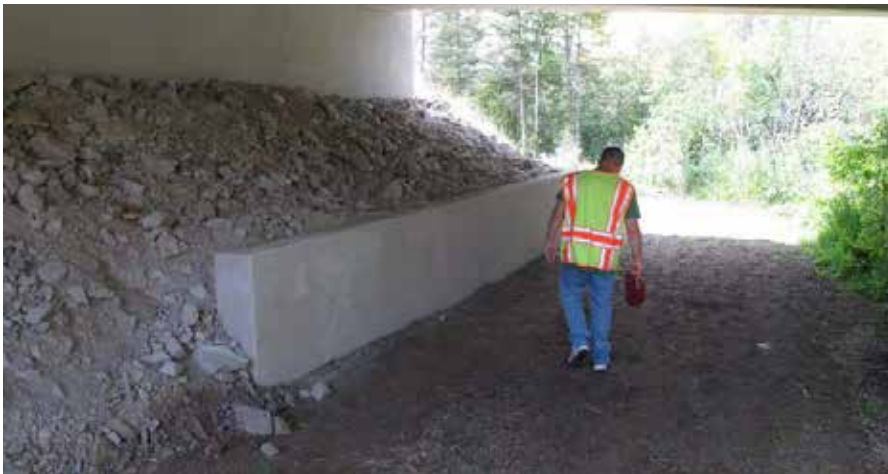
Facilitate movement through wildlife passages by utilizing natural surfacing. The crossing may be coordinated with creek crossings when appropriate. The natural streambank should be maintained through the structure.
